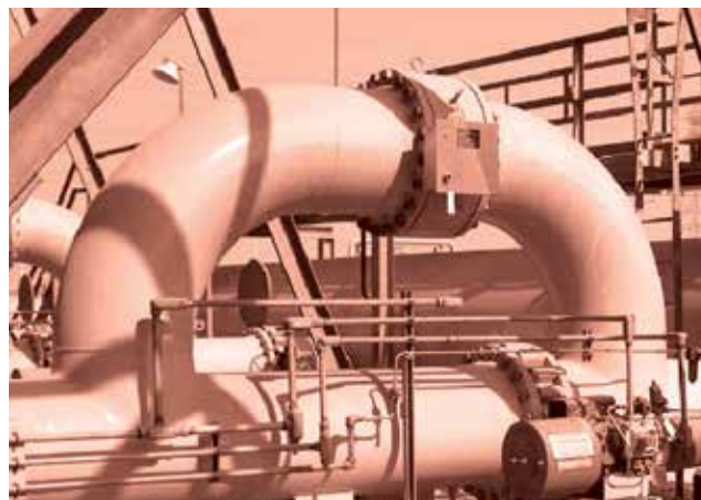
API 537 compliant application
